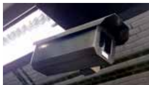
Security and Monitoring
